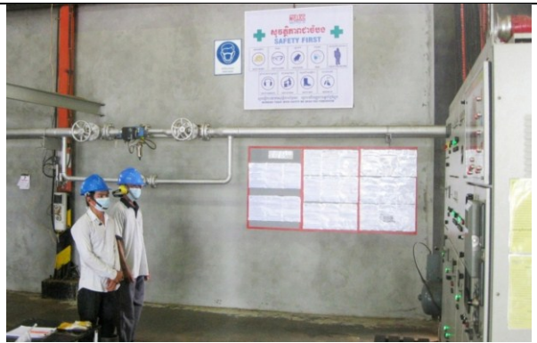
At new POM generator operations, Policy and Procedures displayed available in English and 'Khmer' languages and appropriate PPE worn.
